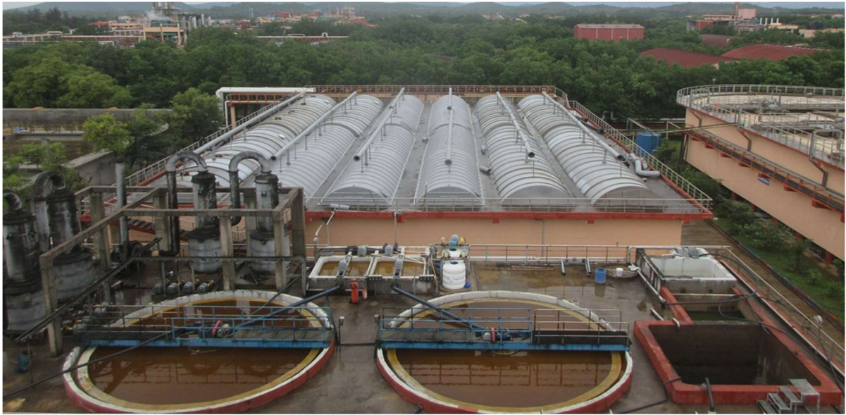
Fig.2.8: HTDS Tanks covered with Hoods and connected to Scrubbers
