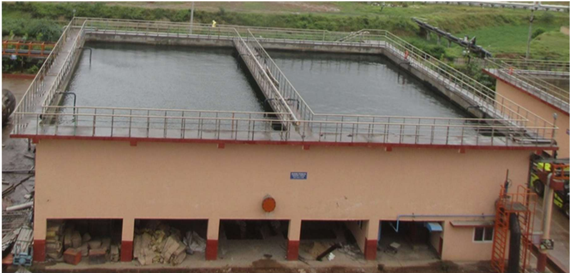
Fig.2.10: Guard ponds for storage of treated Effluent
